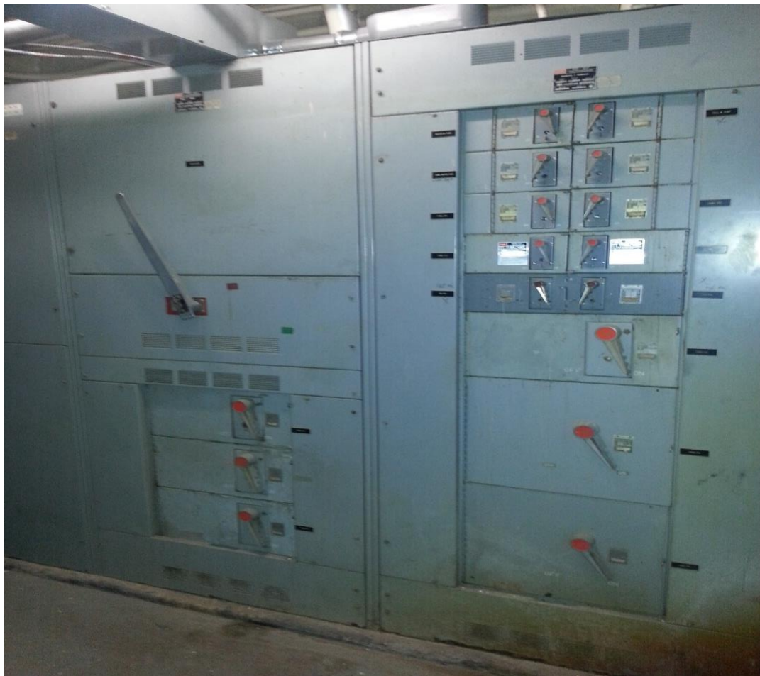
BAB Electrical Service
